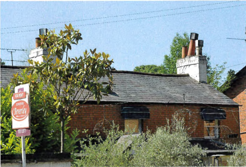
Appendix 10.2 – Chimney stack reset with no cowling
